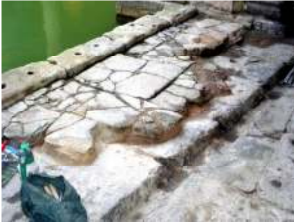
Identifying and specifying repairs to secondary limestone paving in the Great Bath.
