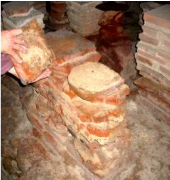
Identifying and specifying rebuilding and rebedding of terracotta pilae stacks, often with the addition of damp proof membranes to slow decay.
