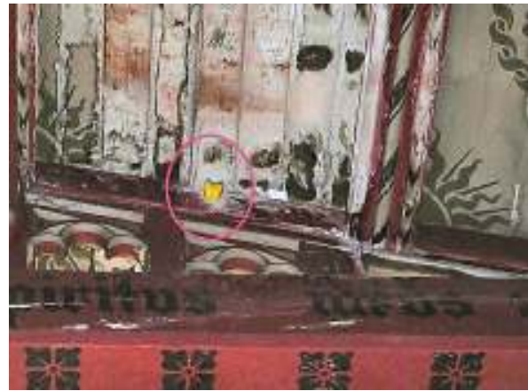
The poor condition of the decorative scheme—a data logger (circled) is installed at ceiling level.
