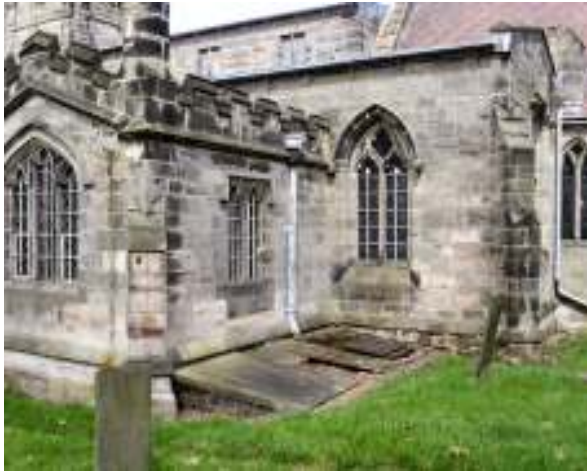
An external view of the chapel, the troublesome shallow pitch lead roof can just be seen
